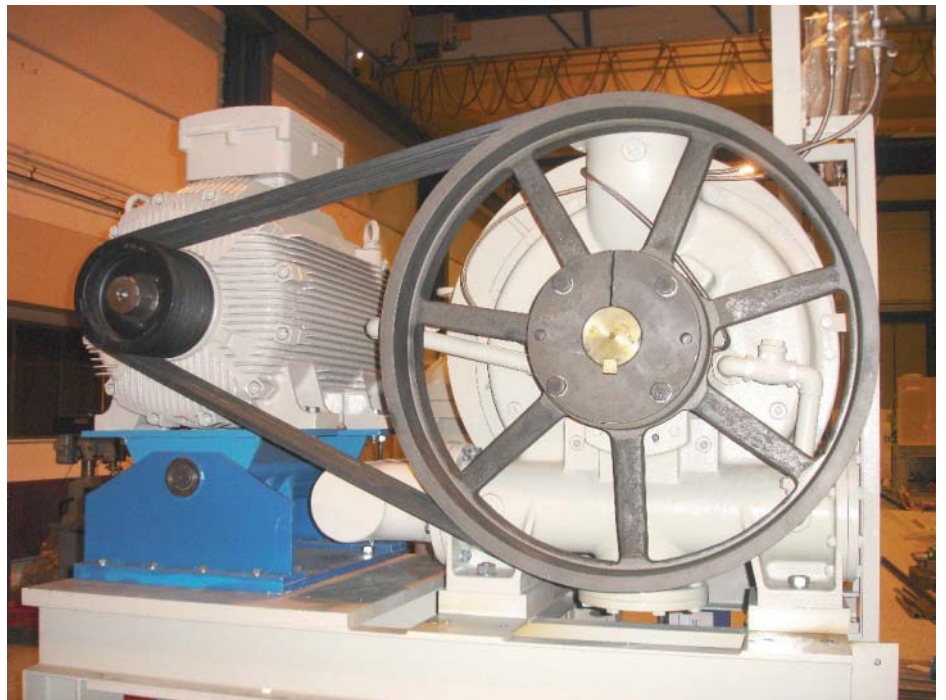
250 kW drive motor for the fluid ring pump on ROSTA Motorbase Type MB 100
